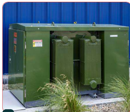
Pad Mounted Transformers
